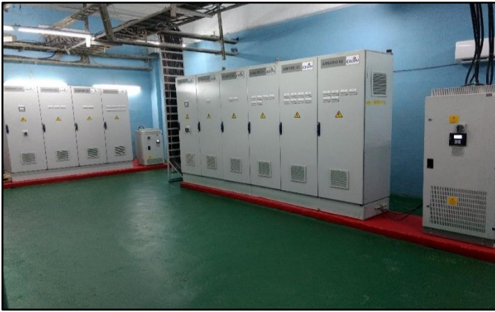
Figure 15: MCC room for wet milling process. Source: Authors, (2020).
