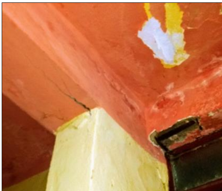
Figure 6: Corrosion caused by the effect of carbonation on the reinforced concrete structure.
