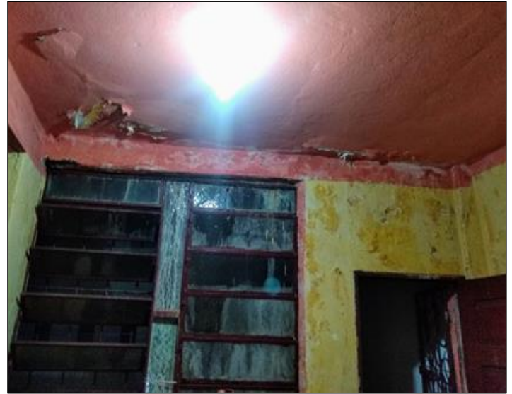
Figure 1: Stains and paint detachment on the kitchen wall of the residence under evaluation. Source: Authors, (2020).
