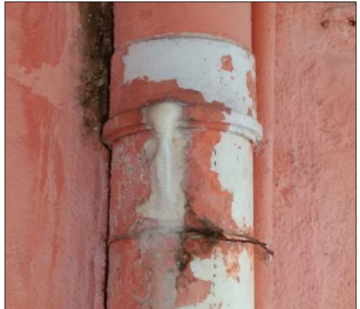
Figure 4: Leaching in the external piping of the service area. Source: Authors, (2020).
