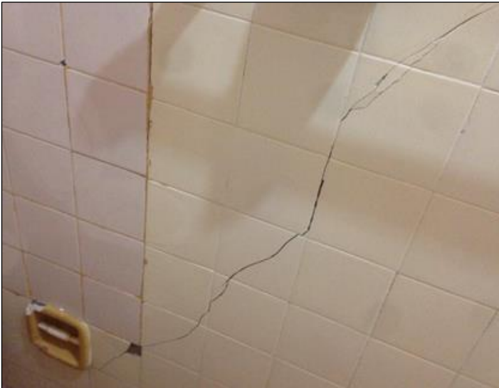
Figure 3: Crack in the bathroom wall caused by repression of the structure.
